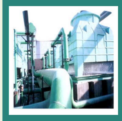
Cooling Water Treatment Chemicals
